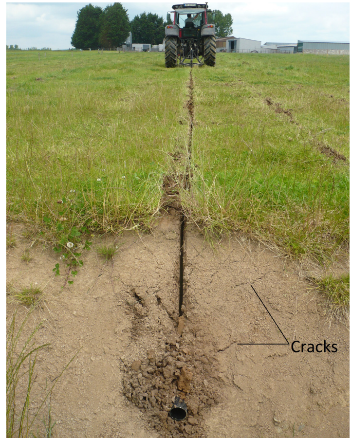
Figure 6- A rigid pipe at the outlet of a mole channel. Notice the soil cracks visible above the outlet (photo credit: Patrick Tuohy).
